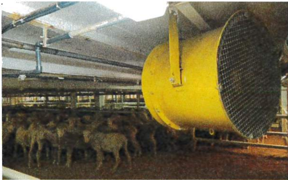
IMG_0109 Large Fixed Fans
