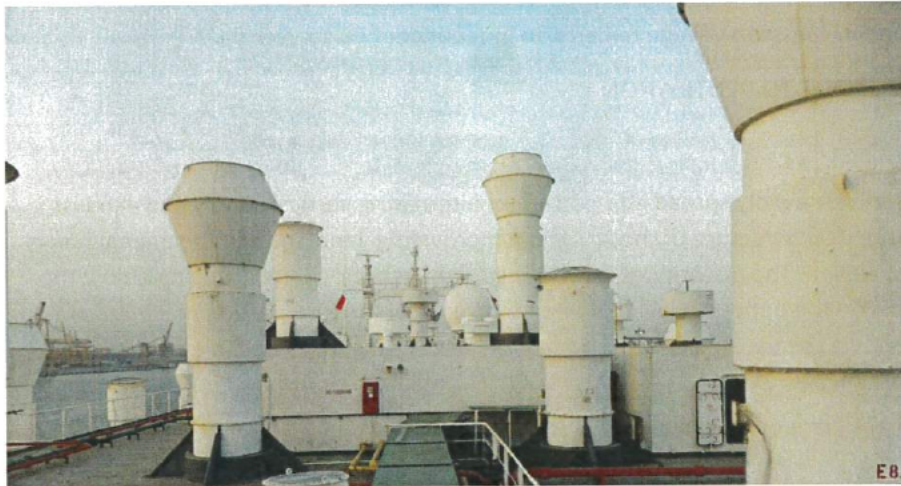
IMG_2089 Conical Exhaust and Flat Top Supply Ventilation Turrets
