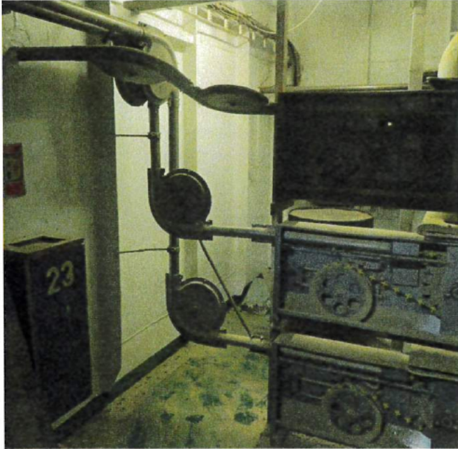
IMG_0740 Feed Lines
