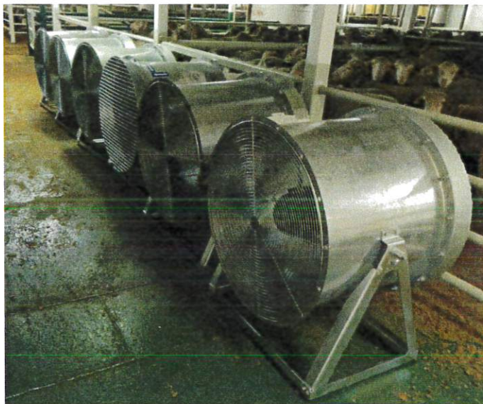
IMG_0161 Six New Fans
