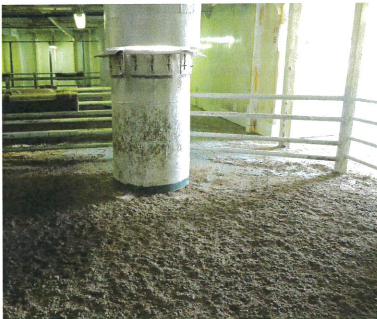
IMG_1581 Differential Drying of the Pad AFT Deck 9, In Pen Supply Vent and AFT Pedestrian Hatch on Right in Image
