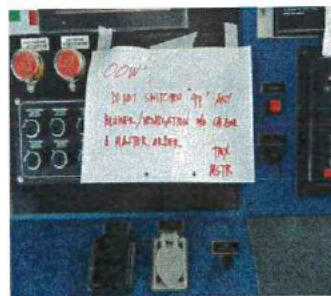
Controls on the Bridge
