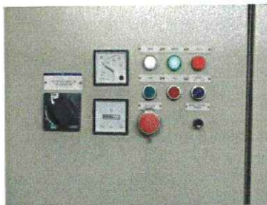
Controls panels found on deck 4
