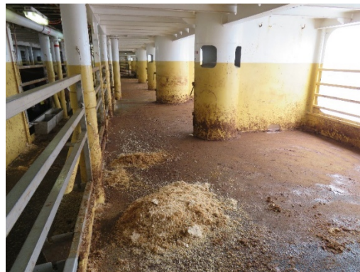
Day 3 Pad drying out after flooding
